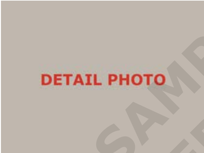
Photo 15. One of three rooftop heating and cooling units.
